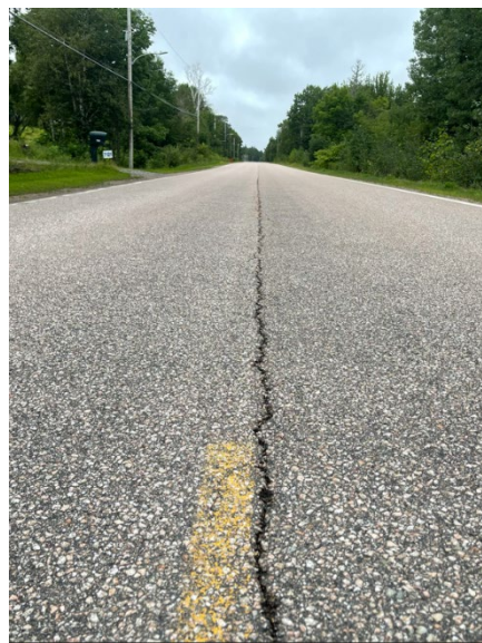
Example of longitudinal cracking
