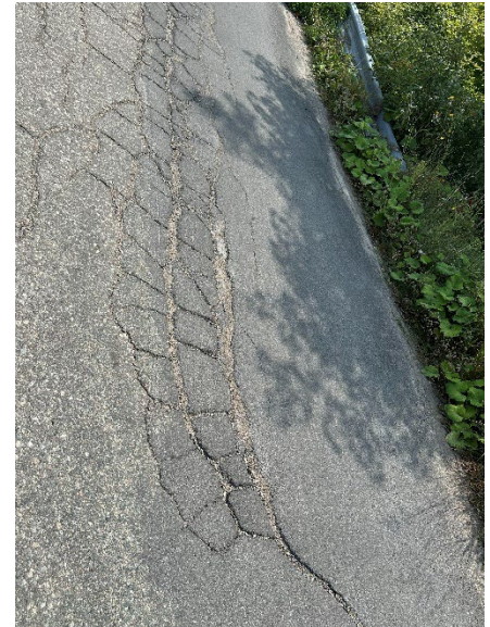
Example of alligator cracking
