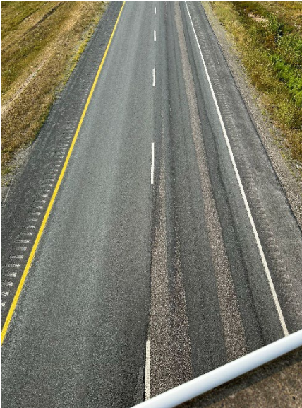
Example of rutting
