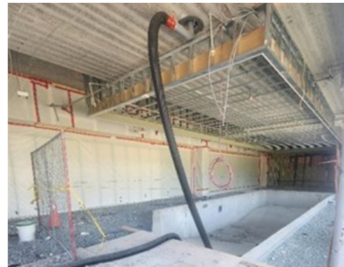
Source: Office of the Auditor General of Nova Scotia – First Floor Pool to be Filled (August 2023)
