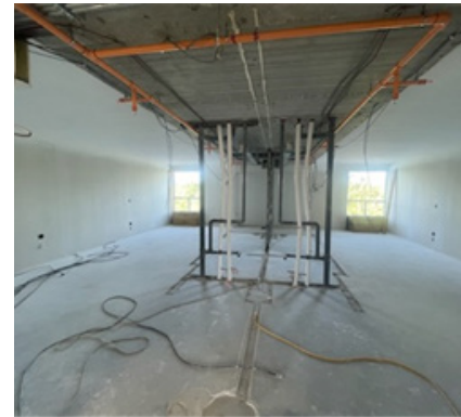
Source: Office of the Auditor General of Nova Scotia – 2nd Floor Renovations (August 2023)
