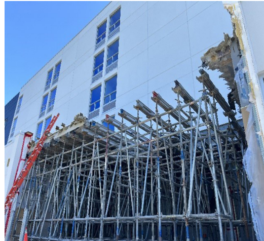
Source: Office of the Auditor General of Nova Scotia – Work to add Additional Stairwell (August 2023)
